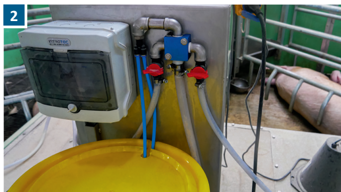
2 Using a circulation pump, the milk is dosed fresh daily and at regular intervals into the mixing container.
